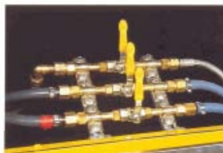
Central manually operated valve control of gases supplied to the machine cutting torches
