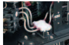
Coated Electrical Connections
